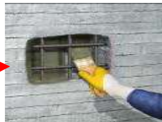
Couche de passivation anticorrosion
