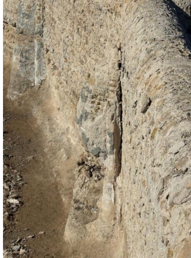
Condition of buttresses showing diagonal cracks.
